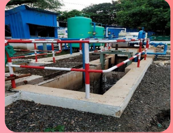
OIL WATER INTERCEPTOR
