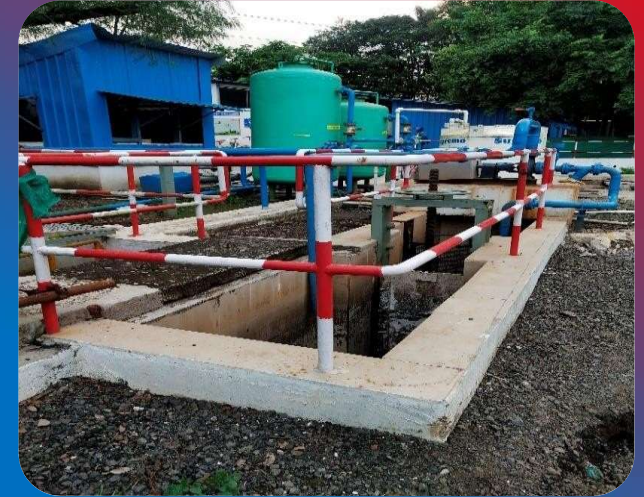
OIL WATER INTERCEPTOR
